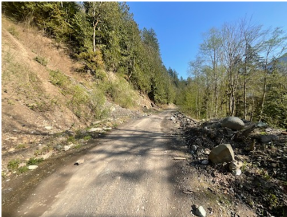
Town approach, unstable upslope and organic wood barrier
