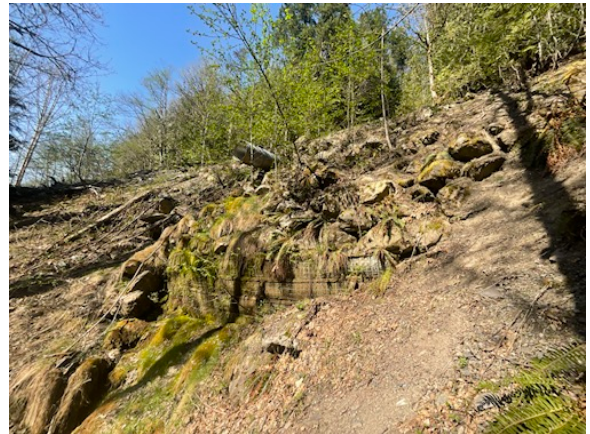
Bulging grs wall under stacked rocks. Seepage and water is somehow getting to culvert.
