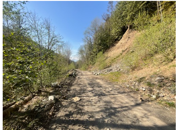
From woods approach. Unstable upslope and no ditch.
