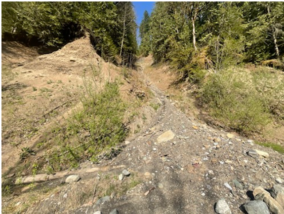
Active landslide upslope. Filled in culvert and ditch.
